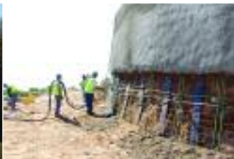
H-beam and lagging system for multistory condo project. Wall installed adjacent to light rail transit line.
