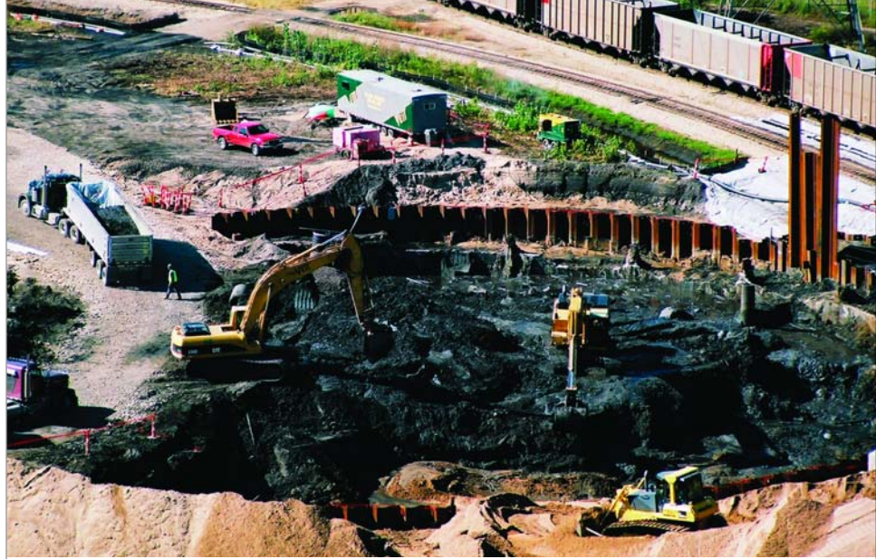
The deep excavation to remove this cyanide contaminated soil required the installation of a sheet pile earth retention system.
