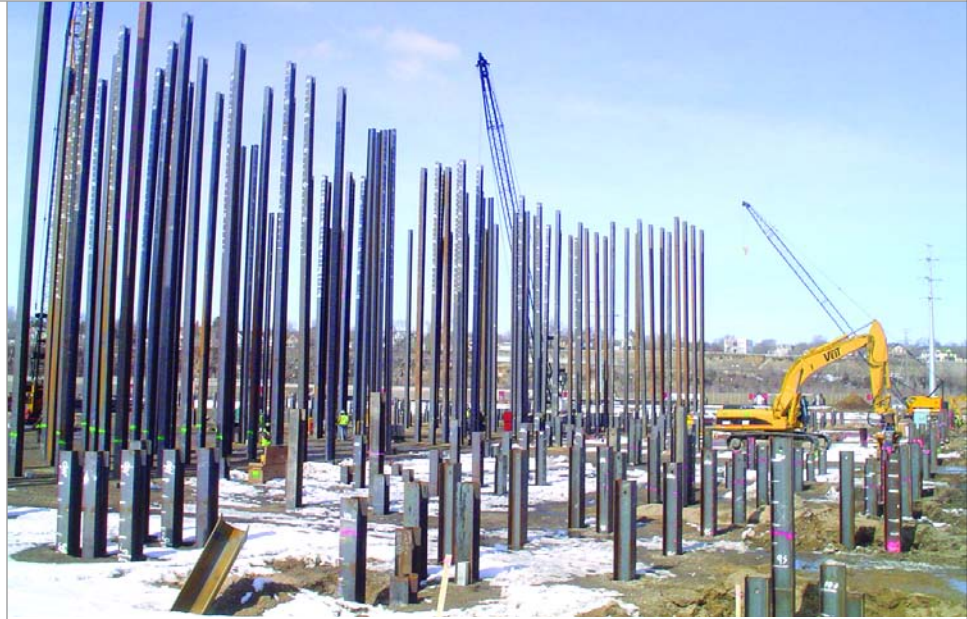
In less than three months, Veit installed 22 miles of H-piles for this power plant project.
