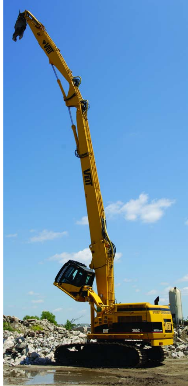
Veit's high-reach backhoe attachment can extend in excess of 125 feet, for quick and controlled high-level demolition.
