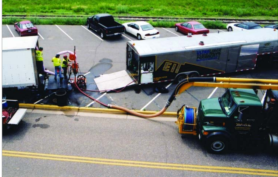
Veit has an excellent safety record for live sewer projects. We work carefully around sensitive utilities.
