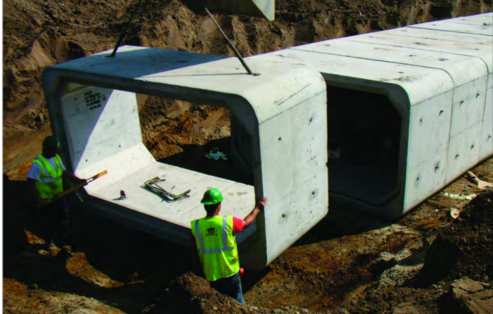
Veit can safely install utilities near highly sensitive areas – and we're just as careful not to disrupt the work of other trades on your project site.
