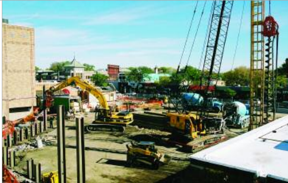
This urban condominium project required five unique foundation/retention systems due to site constraints.
